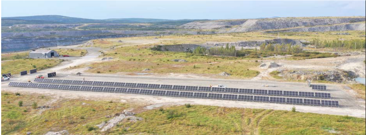
Figure 1. 500 solar panels have been installed, which will be connected to the Troilus camp to provide supplementary and back-up power.
